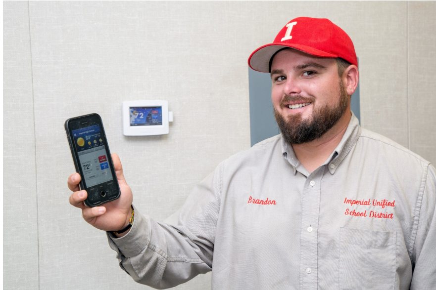
Brandon Machado uses his mobile phone to remotely control ColorTouch thermostats across the district
